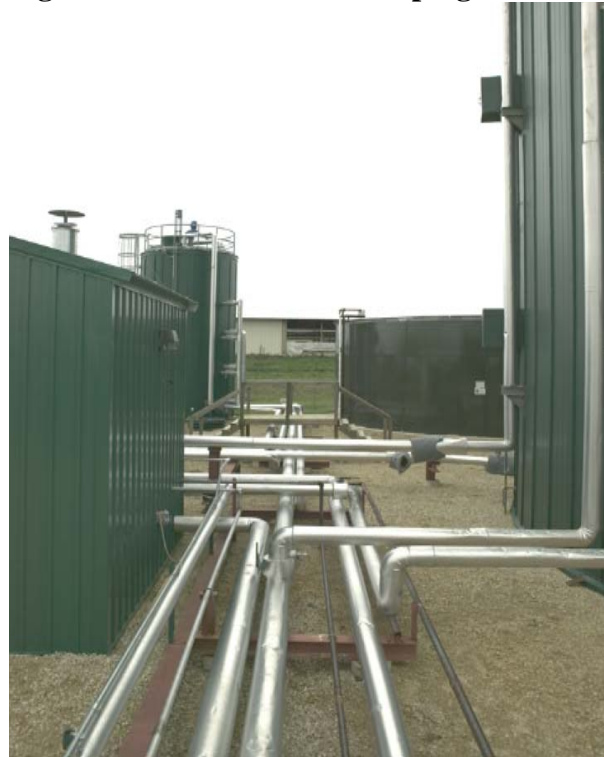
Figure 49 – Structures and Piping at Wild Rose
