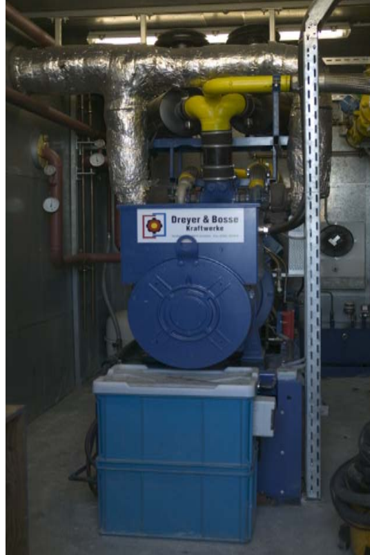
Figure 43 – Suring Engine Generator Set
