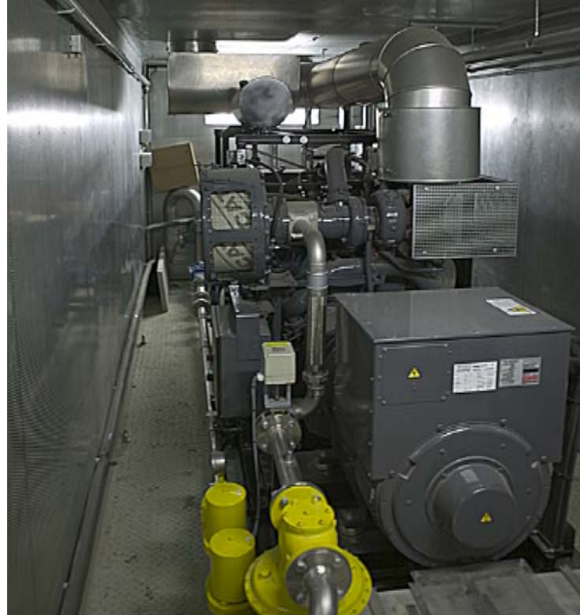
Figure 46 – Engine Generator Set in Container
