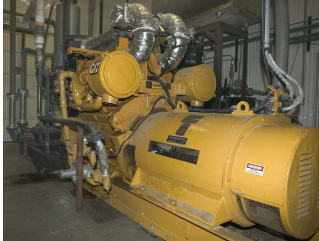
Figure 19 – Double S Dairy Engine Generator Set
